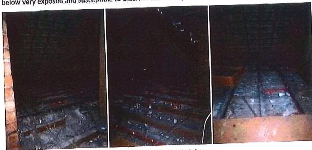
Figure 1 - No Insulation in the loft space.
